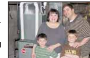
AFTER - Rob, Gretchen, Grant & Foster Johnson w/their BRAND NEW smaller, high-efficiency 90+ Rheem gas furnace.
