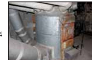
BEFORE - An old gravity furnace converted from coal to natural gas
